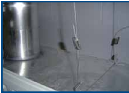
Air conditioning unit
