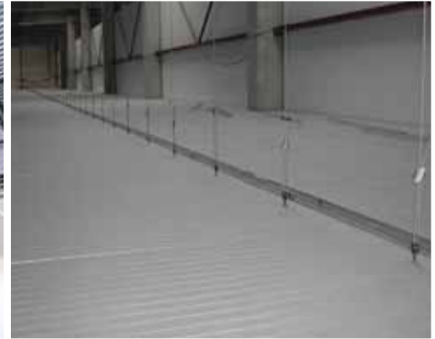
Under panel lighting
