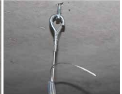
Hook in concrete ceiling anchor
