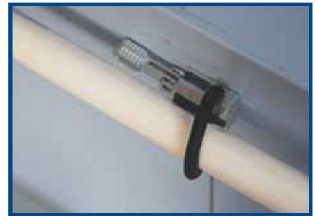
Waste water distribution pipes
