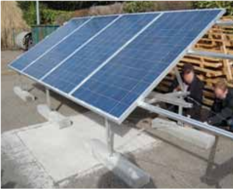
Solar panel bracing
