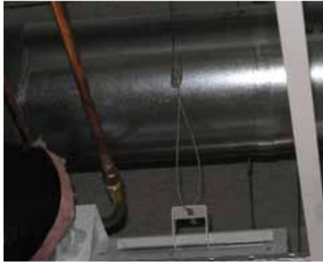
Hangers attached to brackets
