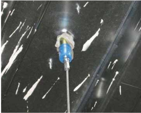
Stud in concrete insert
