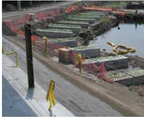
Perimeter safety cables
